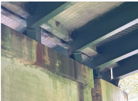
Project #24076 – Bearing Failure
