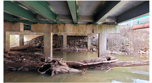
Project #23002 – Snapfinger Pier Caps To Be Replaced
